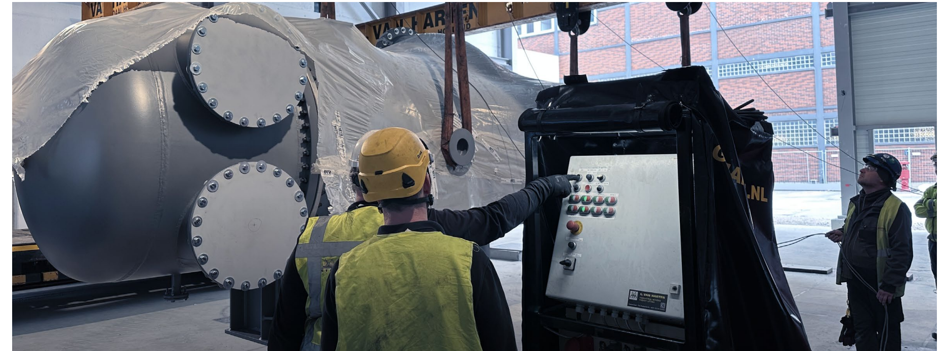
20 MW industrial heat pump for district heating in Mannheim. Image, courtesy Siemens
