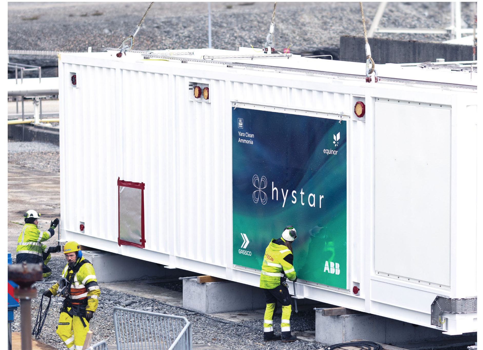
Hystar's "HyPilot" electrolyser being installed at K-Lab at Equinor's Kårstø gas processing plant on the west coast of Norway. This highly anticipated field project unites Nordic industry leaders Equinor, Yara, and Gassco as well as ABB. ABB's low-harmonic insulated-gate bipolar transistor (IGBT) rectifiers and DC-DC converters will regulate the supply of electricity to enable the electrolyser to operate under realistic field conditions. ABB will provide local support and expertise on the ground in Norway throughout the project's duration. Operators will gather data during the 10,000-hour trial to demonstrate that green hydrogen can be produced cost-effectively and reliably by utilizing renewable energy sources, such as wind power. Image, courtesy Hystar
